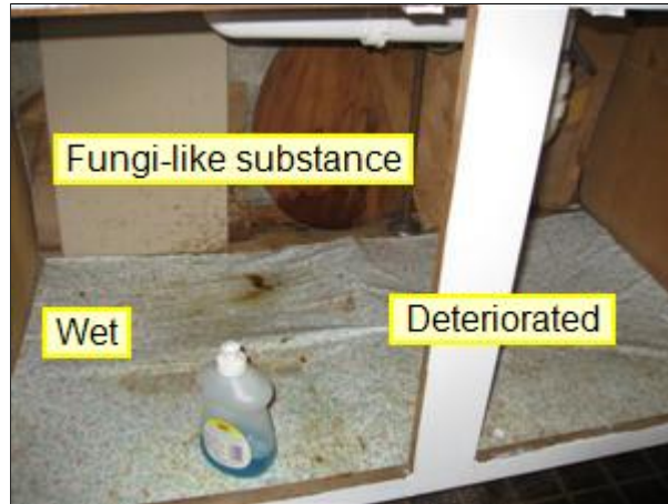
3.4 Picture 1 under kitchen sink
