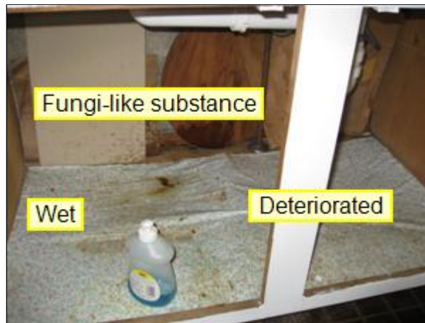
3.4 Picture 1 under kitchen sink
